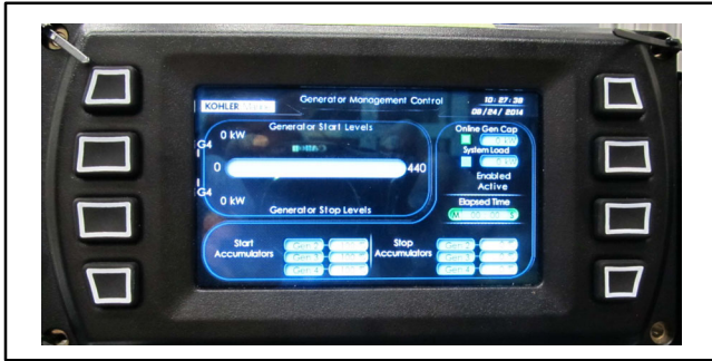
Figure 26 Generator Management Screen
